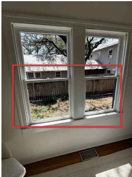
Painted shut bedroom windows still present
