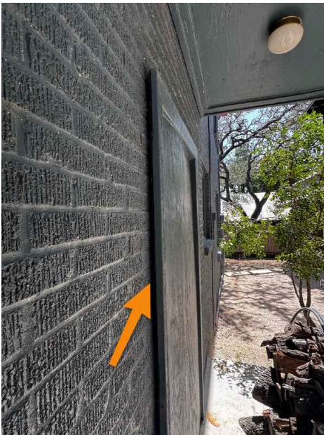
Improper sealing at backside
