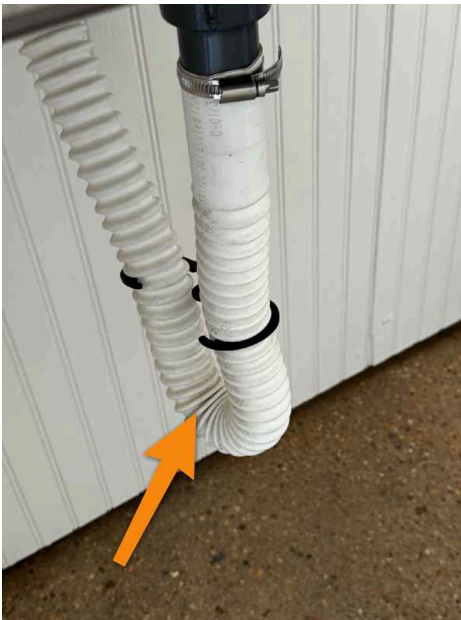
Missing P Trap exterior bath
